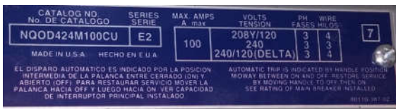
B.O.H. ELECTRICAL PANEL AND LABEL UPPER LEVEL
