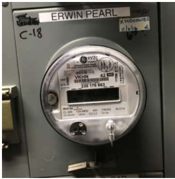
TERMINAL 3 CONCOURSE HK APEX ELECTRICAL METER
